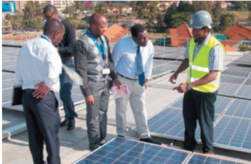
ERC staff on a tour of a solar photovoltaic (Solar PV) installation used to generate electricity.
