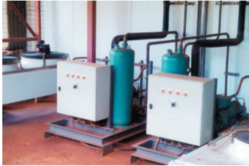
Compressed Air System. One of the systems analyzed during audits in a factory that uses compressed air.
